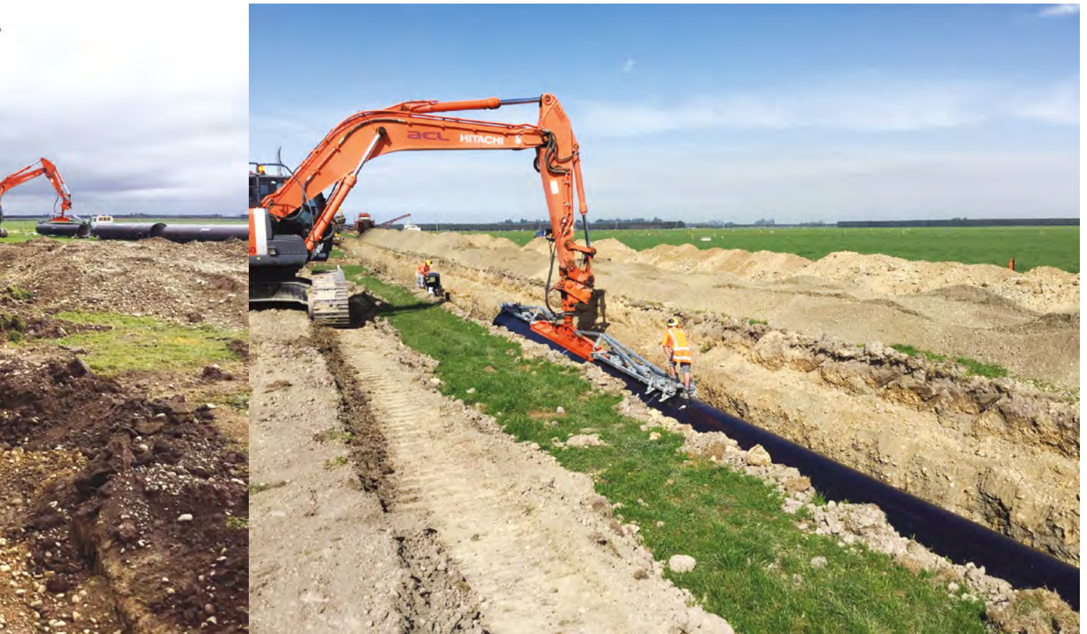
Ashburton-Lyndhurst Irrigation Scheme laying the main pipe for delivering irrigation water under pressure
